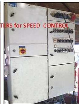
Main electric centre
